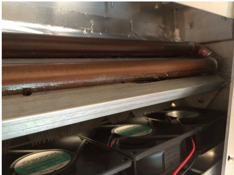
Fig 13: Fans and heat exchanger at the top of the unit.
