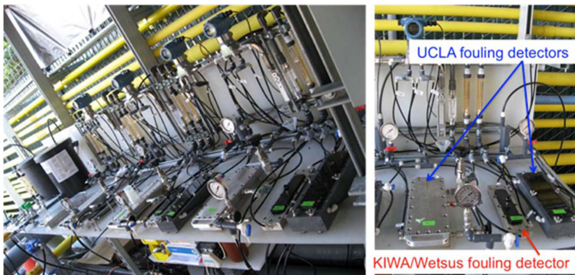
Fig. 11 Pictures of various fouling detectors employed at a seawater desalination plant. Research conducted at the Long Beach Water Department's seawater RO/NF demonstration plant focusing on NF/RO membrane biofouling mechanisms, prevention, and monitoring. Tanuwidjaja 107 compared three different membrane fouling detectors to understand potential bias due to different monitoring device configurations. At left, four parallel trains of 3 sensors per train are depicted. At right, a single train of 3 fouling detectors including UCLA's high-pressure fouling detector, which enables flux, rejection and differential pressure to be monitored as well as a UCLA low-pressure fouling detector and a KIWA/Wetsus low-pressure fouling detector; both low-pressure fouling detectors monitor differential pressure only. Original image courtesy of Dian Tanuwidjaja. Copyright University of California, Los Angeles.
