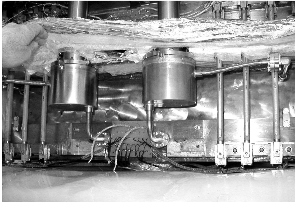
FIGURE 5. Condensers attached to cryocoolers. The upper (vapor) and lower (liquid) lines are shown. Also shown are several of the high T_c current leads
