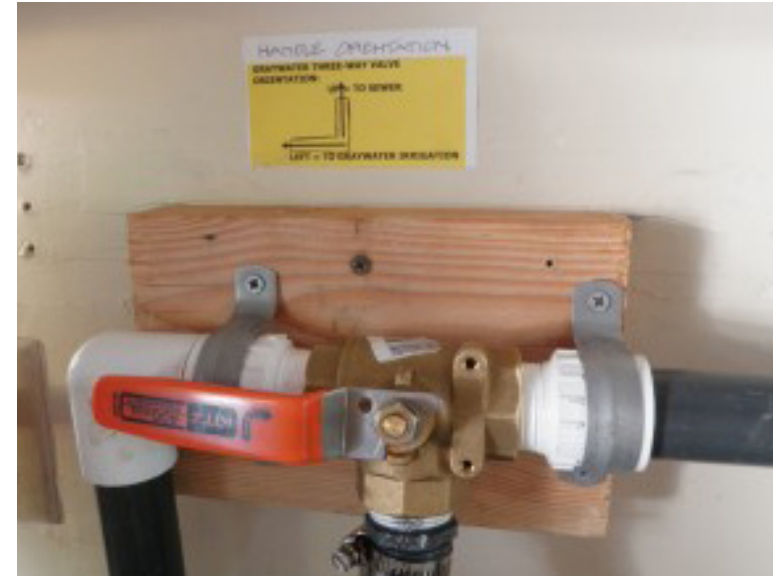
Laundry to landscape graywater system 3-way valve separates water destined for the sewer from water used to irrigate landscape plants. Photo: Central Coast Greywater Alliance
