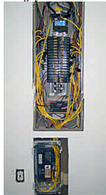
Eaton Cutler-Hammer Panel
