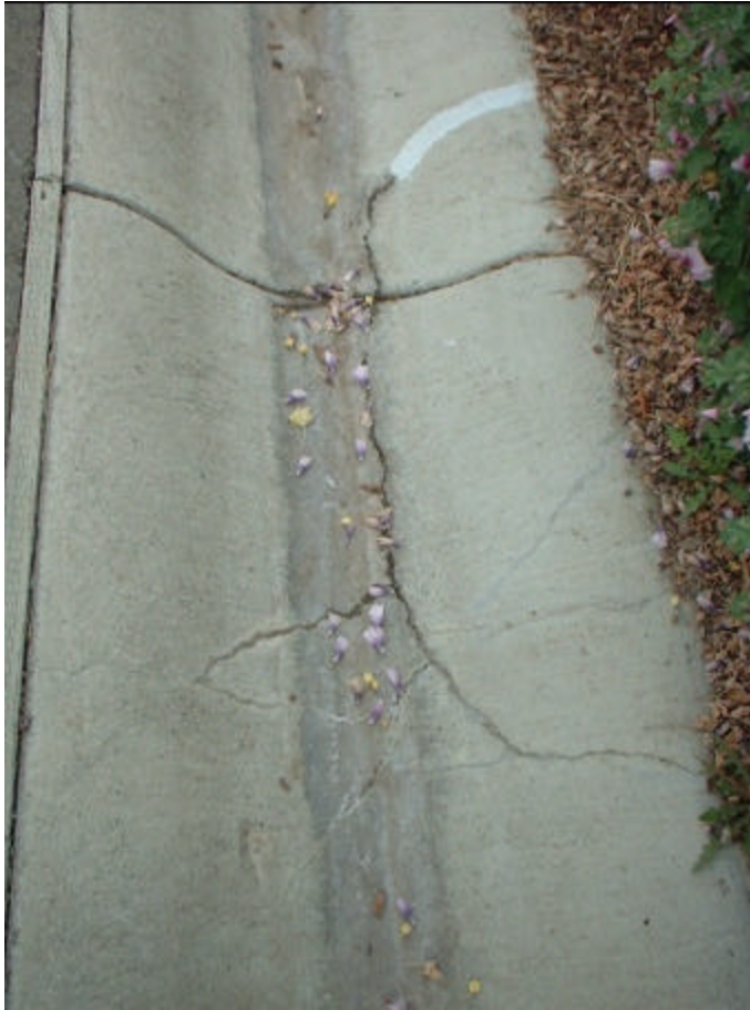
Figure 3: Cracks in V-ditch at Tassajara Creek, 3/25/2004
