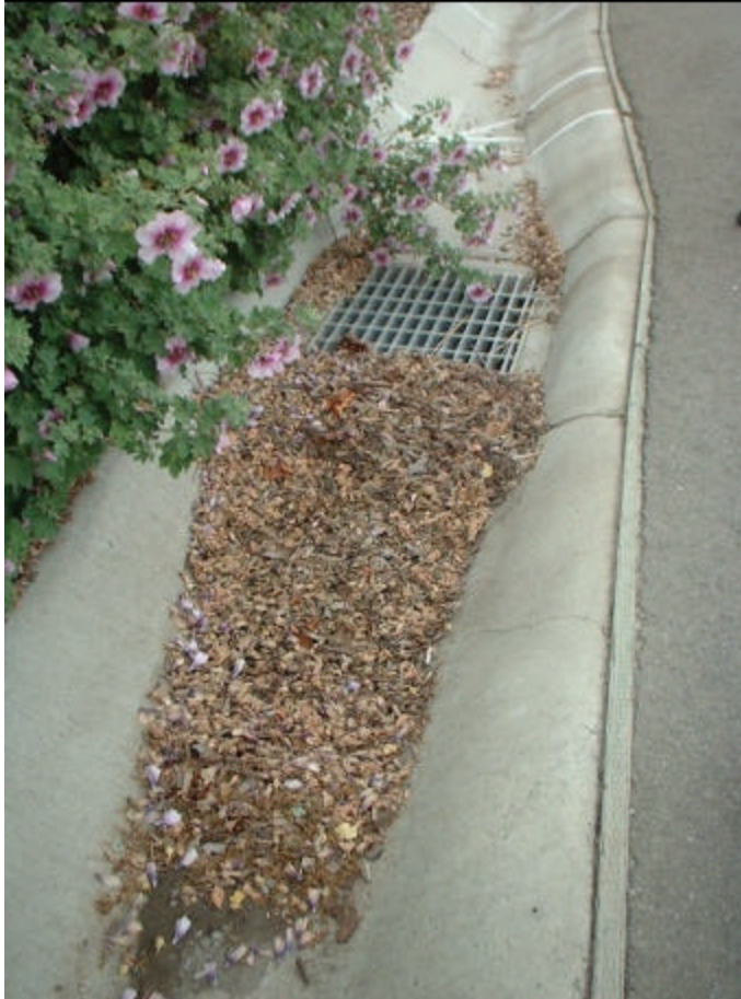
Figure 4: Debris clogging a drainage grate at Tassajara Creek, 3/25/2004
