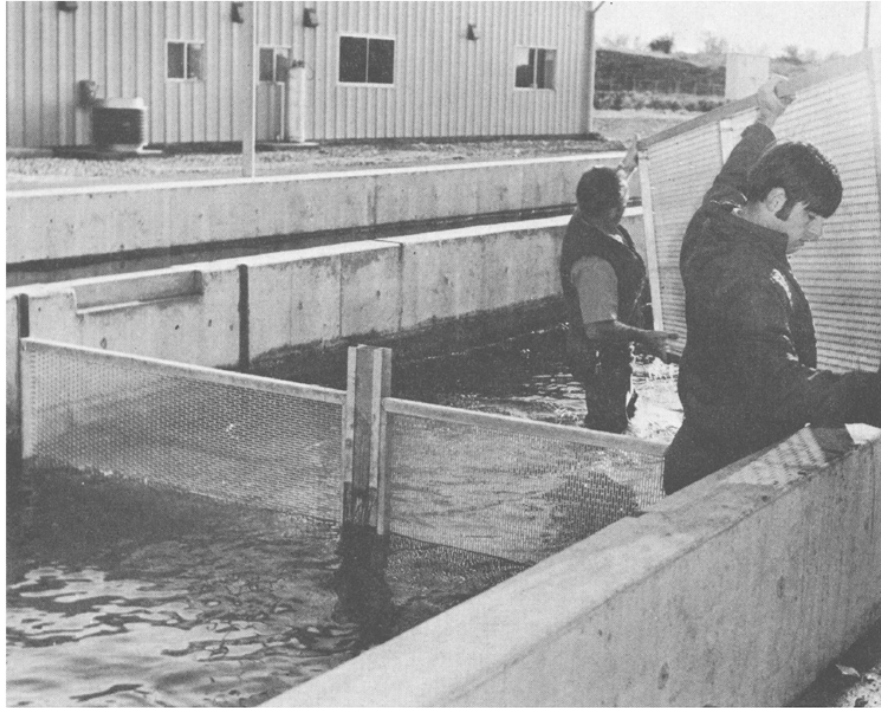
FIGURE 48—Concrete rearing ponds are 10 feet in width with keyways in the concrete walls for screens and checkboards. Note metal removable post that fits in a pocket in the concrete floor so two 5 foot screens can be used instead of one long screen. Photograph by George Bruley, 1973.
