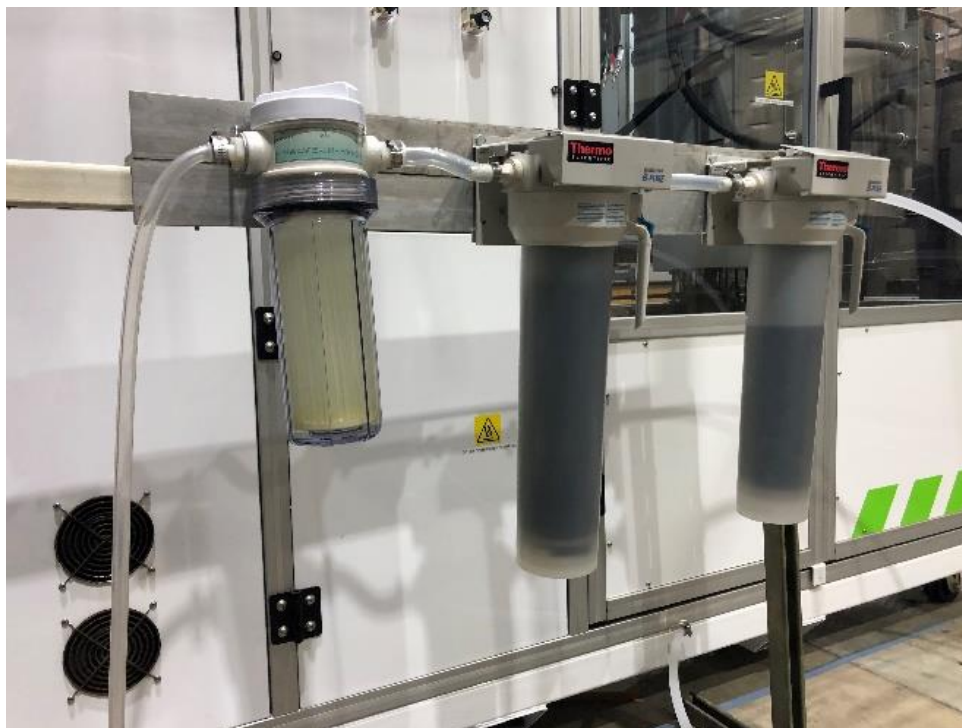
Figure 74: Deionized water supply line.
