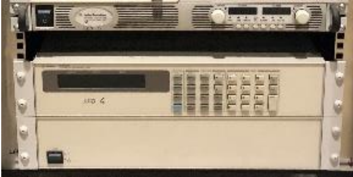
Figure 72: Electronic load and power supply.
