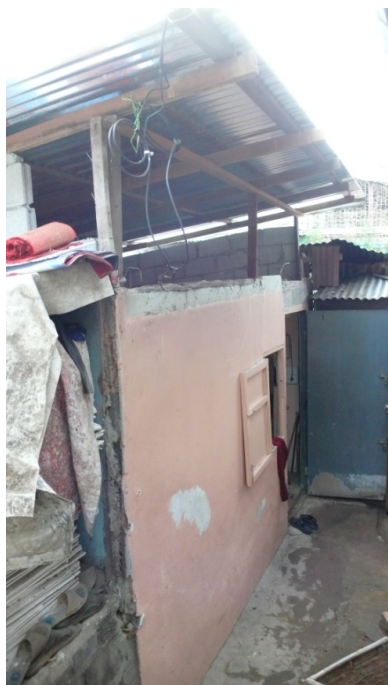
Figure 5.11: An upgrade left unfinished due to insufficient funding. Source: N/A
