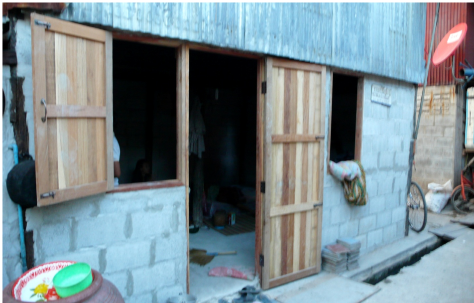
Figure 5.10: New doors, concrete bricks, and corrugated metal purchased with CODI upgrade grants and private loan money. Source: N/A
