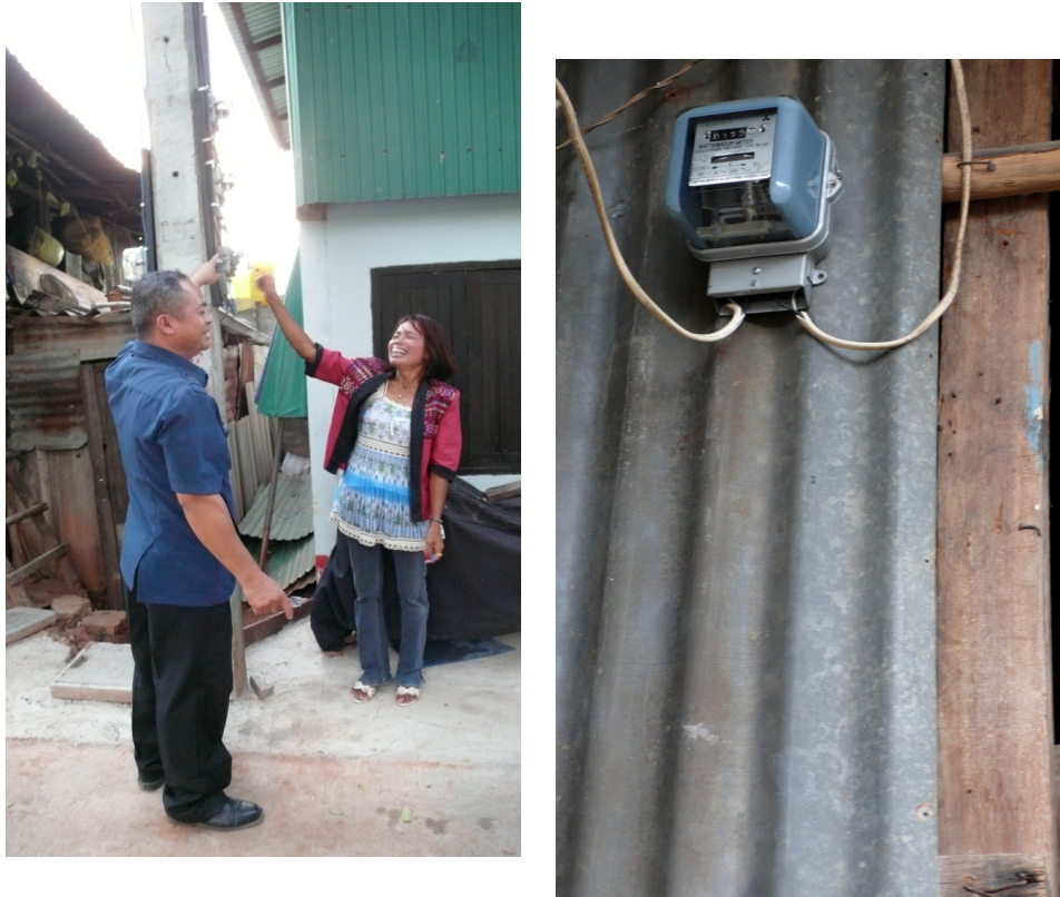
Figure 7.3: Permanent (right) and temporary (left) electric meters.
