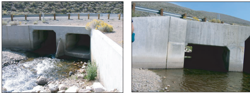
Figure 4. The right culvert chamber has a perched inlet (shown left). Combined with the same culvert's inundated outlet (right), it is difficult for many terrestrial animals to use. Photos S. Jacobson.
