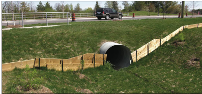
Figure 4. Dry culvert at McKenzie Wetland with drift fencing to direct wildlife movement.
