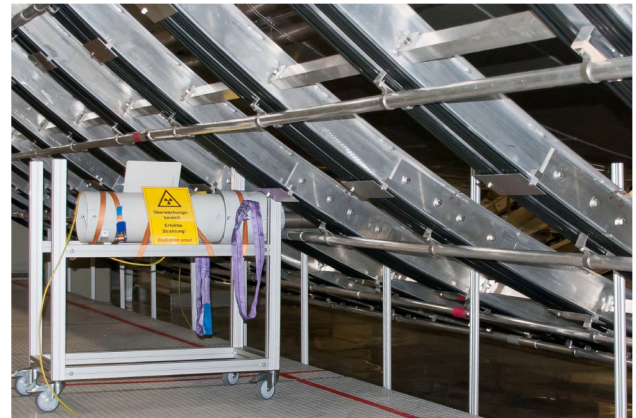
Fig. 5 The ^{60}\text{Co} source used to increase the gamma radiation at the MS. The upper panel is a schematic of the source (in the “closed” configuration). In the bottom panel, the source can be seen installed next to the air-coils, beneath the MS vessel
