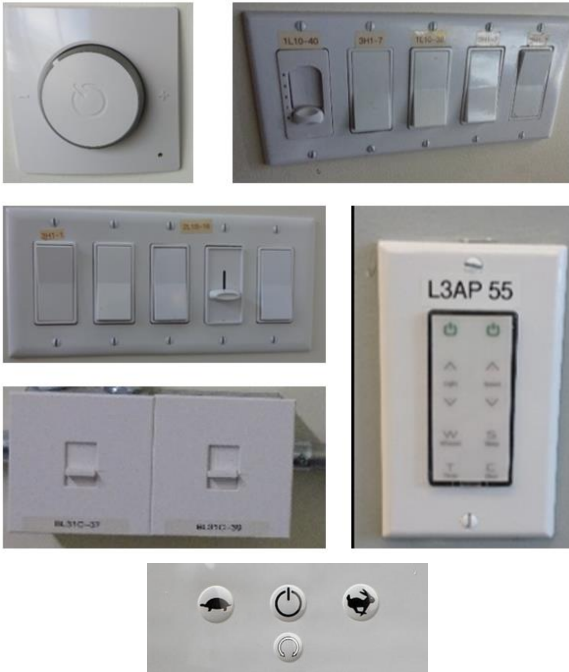
Figure 32: Examples of ceiling fan wall controls (Images courtesy Elaina Present)
