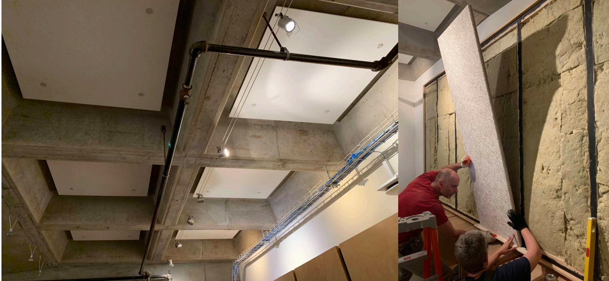
Figure 3: Views of completed ceiling treatment (left) and installation of the treatment along the east wall (right).
