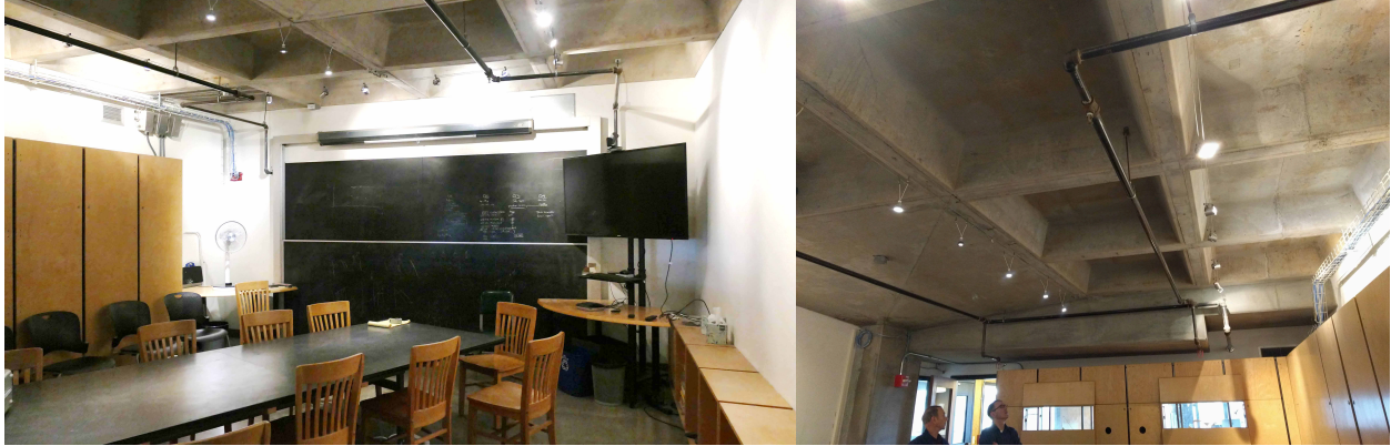
Figure 1: Room 390 as found in 2018. The walls are all hard surfaces and the ceiling is exposed concrete. The room has an RT60 of 0.82 seconds in the speech frequency range, thereby exceeding the target value of 0.6 seconds. The reverberant characteristics of Room 390 make it challenging to understand speech, especially during teleconferences.
