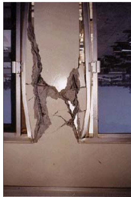
(b) Interior up-close view of the column damage caused by the earthquake
