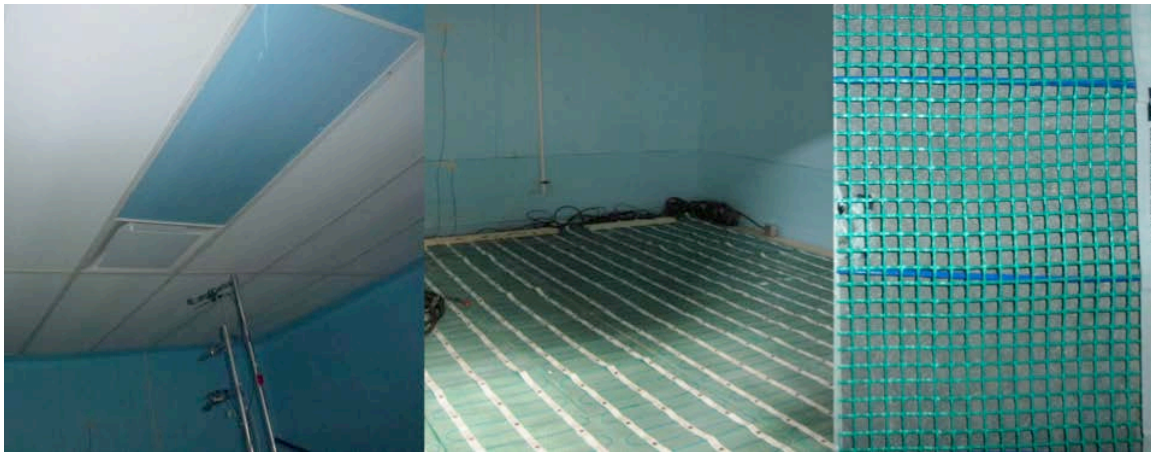
Figure 4-2: (a) Radiant ceiling configured to have air diffuser in the middle for air system test, (b) floor heating mats on top of concrete boards, (c) porous feature of the heaters allowed heat transfer between concrete and the rest the room
