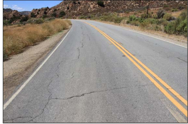
Figure 2.4: Block crack progression.
