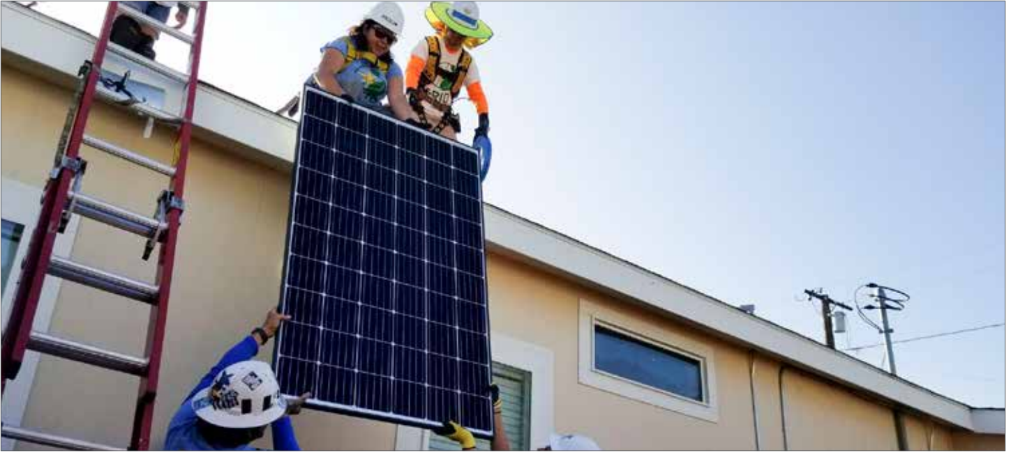
GRID Alternatives staff and trainees install rooftop solar photovoltaic panels in July 2019. Photo credit: GRID Alternatives
