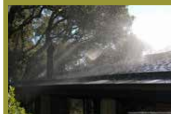
Photo 1. Roof mounted sprinkler.
