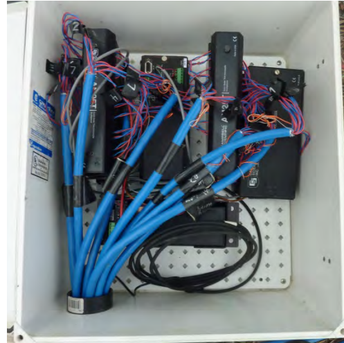
(b) Data collection system (inside)
