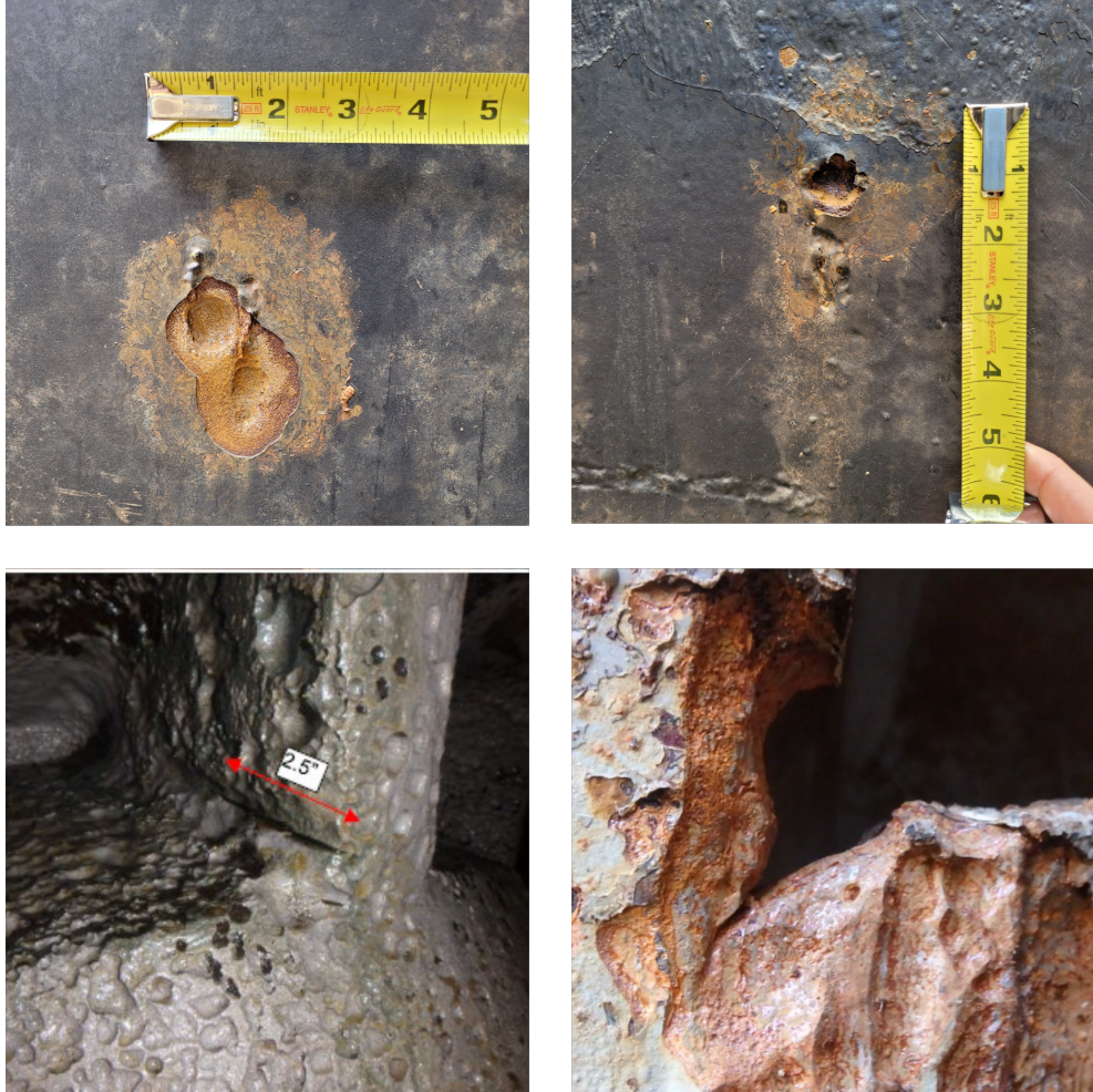
Figure 5.1. Pitting corrosion images on miter gates [77] (Courtesy of Brian Eick)
