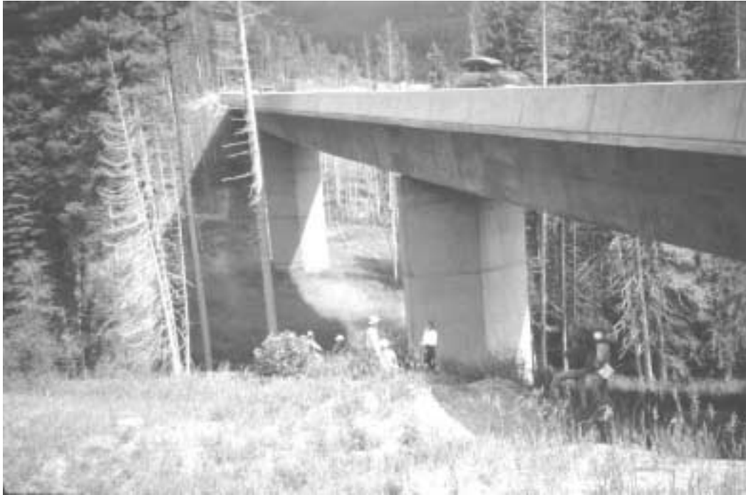
Fig. 1. Span on I-70 in Colorado, east of Vail. Structure has grasses and other vegetation. Light transmission is excellent and avoidance by most mobile species would be low.
