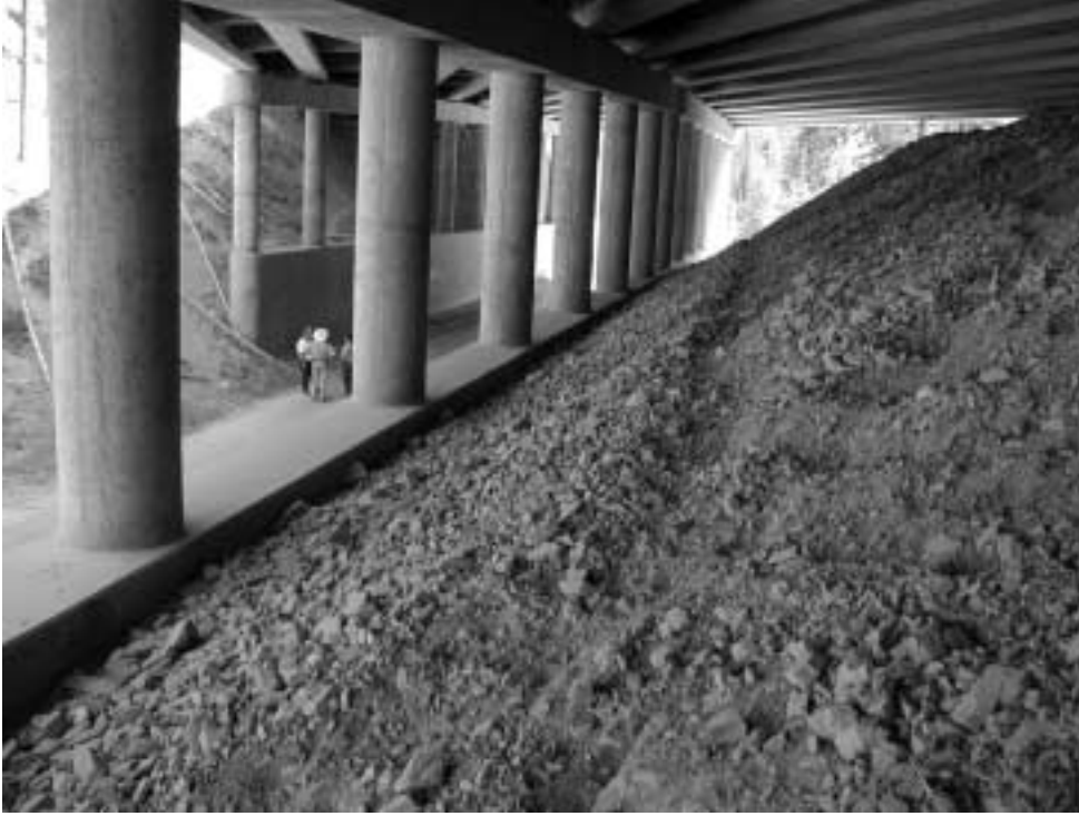
Fig. 4. Indicates a deer trail in the foreground. Deer and other animals used this portion of the bridge rather than the road surface.
