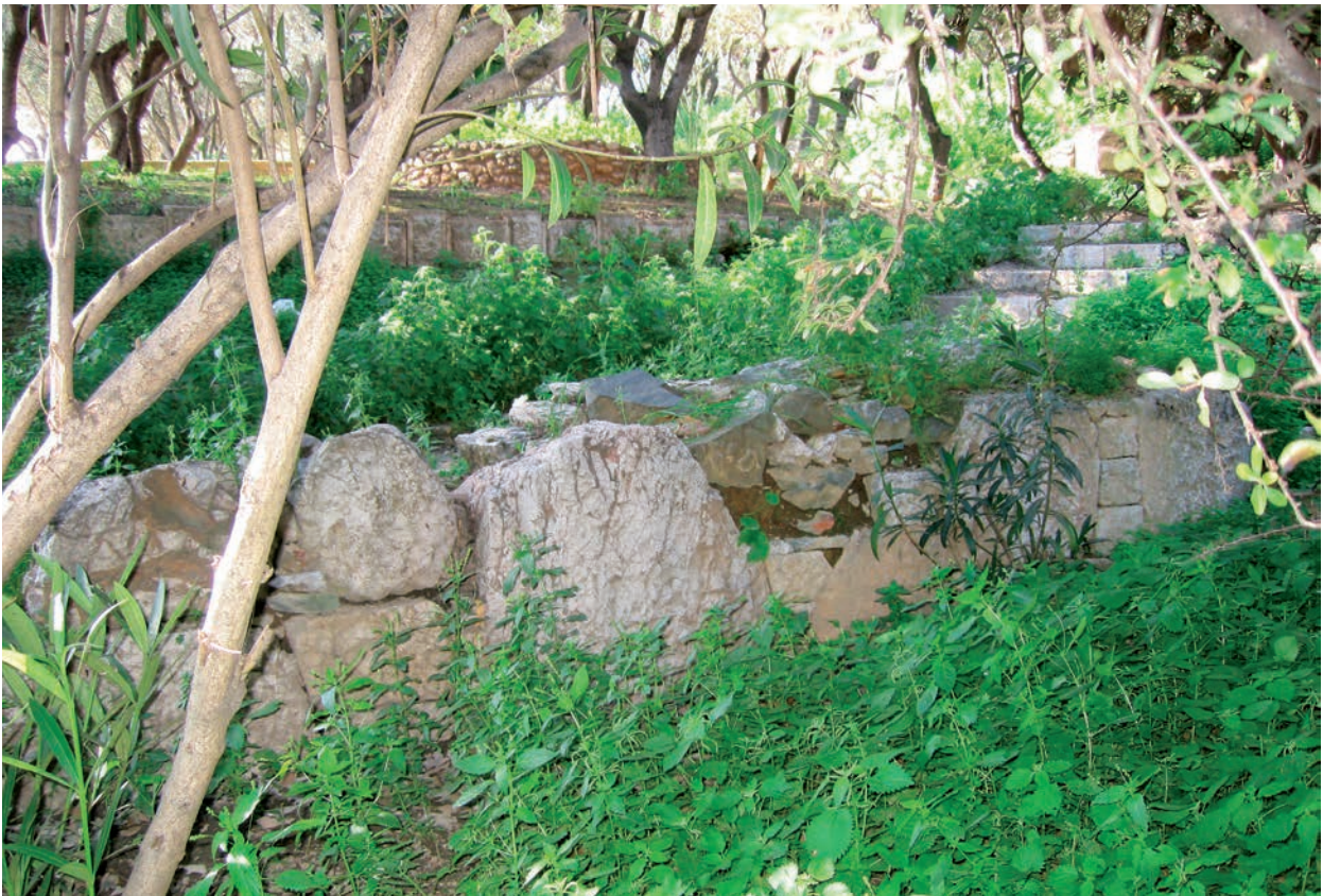
Figure 4.1. Athens, Acropolis. South Slope, south of the Herodeion. Retaining Wall 162. Photo by Eirini Dimitriadou, 2010.
