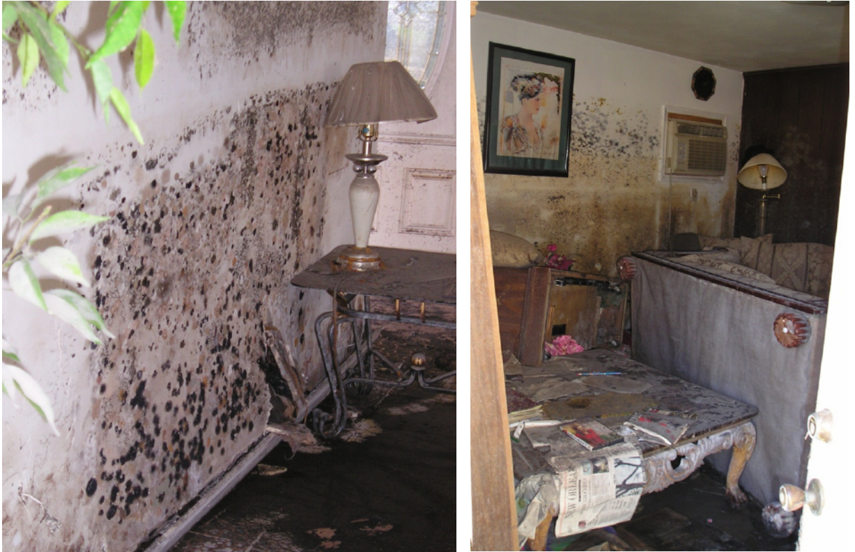
FIGURE 3.1.5 Flooded homes after Hurricane Katrina, New Orleans, 2005. Photographs by Gina Solomon.
