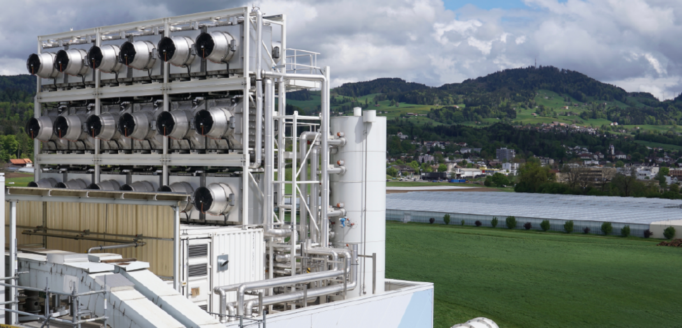
FIGURE 18.2.6 The Climeworks direct air capture facility near Zurich, Switzerland, uses 18 modular capture units to remove \text{CO}_2 from the air. The purified \text{CO}_2 is then used to enhance the growth of vegetables in the greenhouses in the background—not really negative emissions yet, but a demonstration of the costs and issues associated with separating \text{CO}_2 from air. This facility catches about 1,000 tons of \text{CO}_2 per year. Photograph by Roger Aines.
