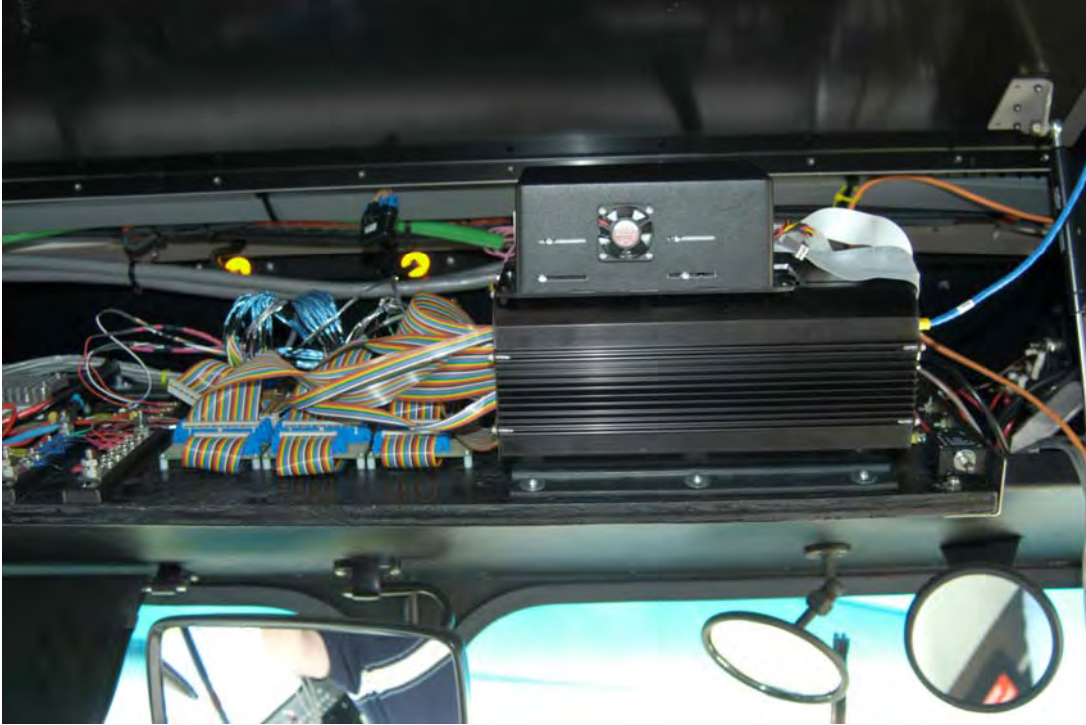
Figure 3.2.5. PC/104 Control Computer Installed in New Flyer Transit Bus.
