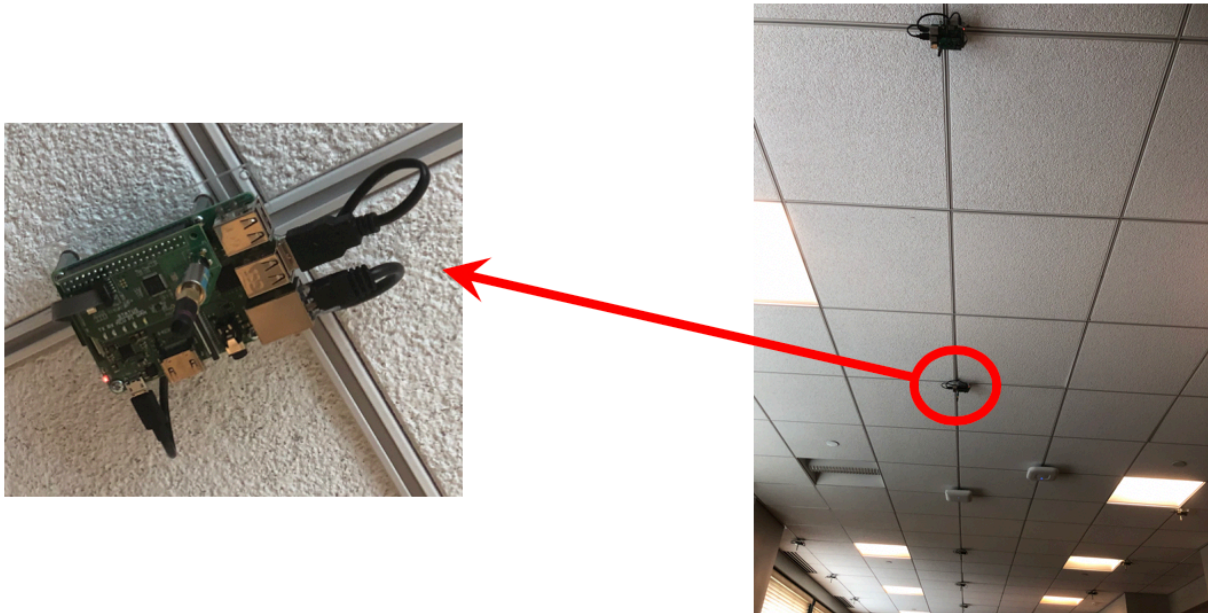
Figure 63: Hamilton Border Routers installed in ceiling in office in Soda Hall, UC Berkeley.
