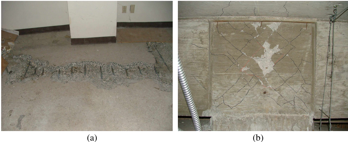
Figure 2. Earthquake damages of the building, (a) Punching shear failure (Column B6 at the 3rd floor level), and (b) Shear crack on beam-column joint (Column A4 at the 3rd floor level)
