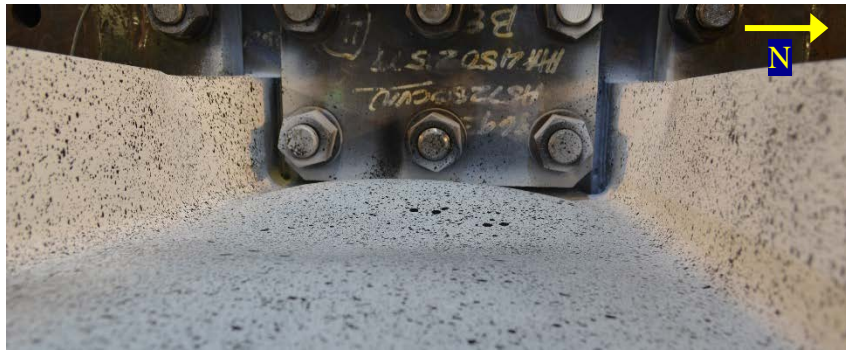
(c) Web Local Buckling at West End
