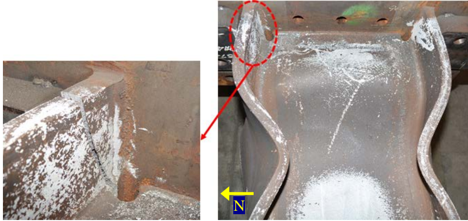
Figure 4.4 Specimen 11M: Column Fracture at End of Test (Northeast Flange)
