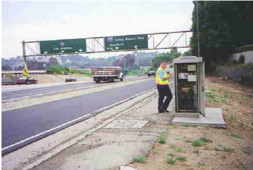
Figure 4.4: Cabinet location next to freeway.
