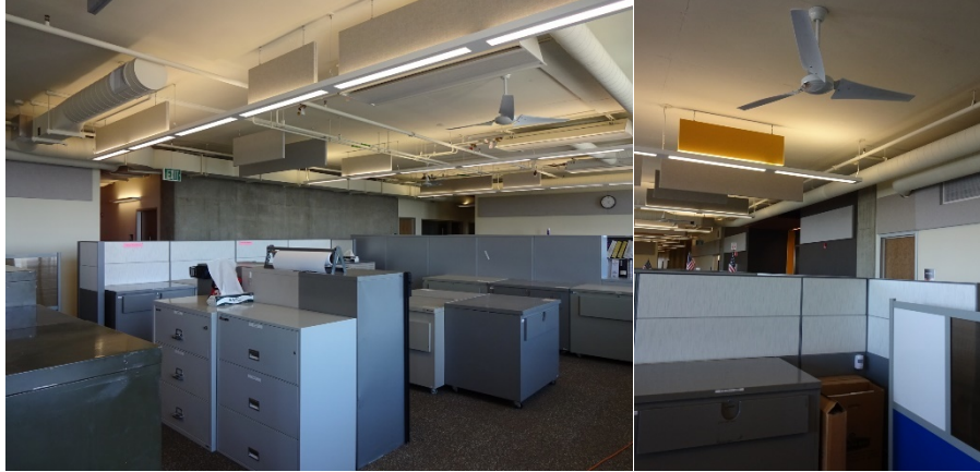
Figure 5-9: Typical open plan office space with TABS radiant ceiling, ventilation ducts, acoustical baffles, and ceiling fans.
