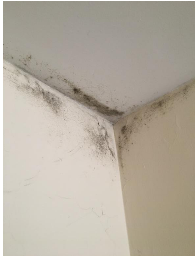
Figure 10. The mold in the corner of Mary’s living room in Brimstone House (Carolina Talavera)
