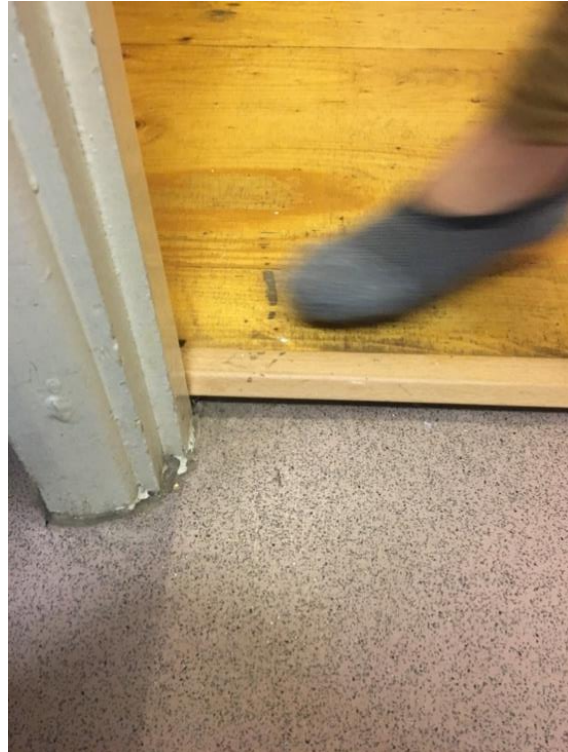
Figure 3. One of the girls uses her foot to show me the gap in the floor between the bathroom and the hallway where she said spiders and cockroaches entered the flat (Carolina Talavera)
