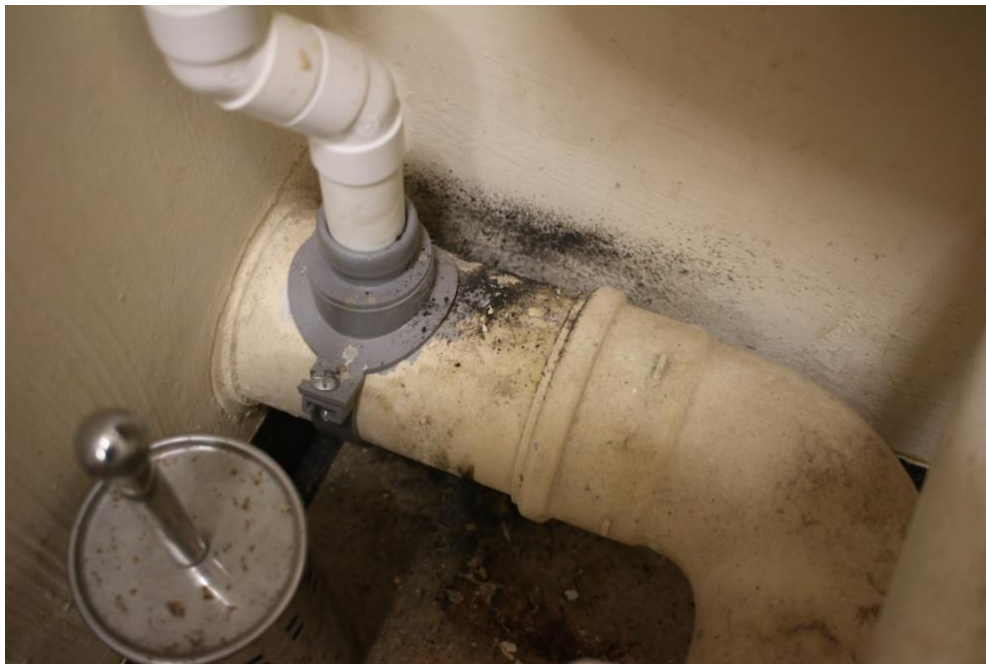
Figure 8. Mold behind the toilet and on the pipes (Carolina Talavera)
