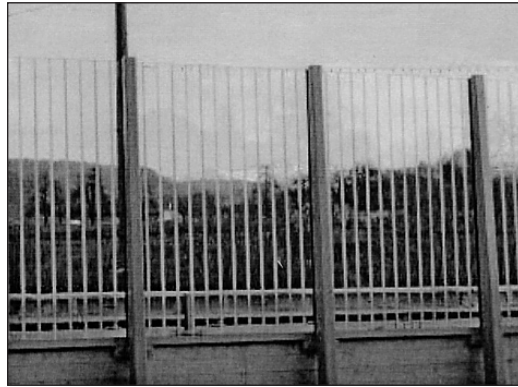
Figure 14. Example of a transparent noise barrier with a striped pattern as recommended by Schmid & Sierro (2000) to disclose the glass to birds eyes. (Photo courtesy of Joggi Rieder, Kaden und Partner AG)
