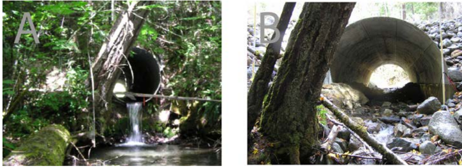
Figure 2. An example of before (A) and after (B) road-stream-crossing reconstruction from STC.
