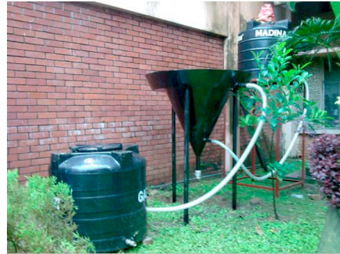
Photograph 6. 100 L/h prototype system temporarily installed at BUET for testing.
