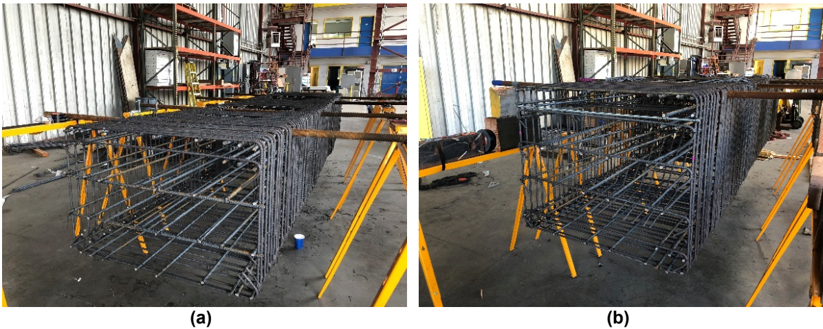
Figure 6.17 (a) Completed foundation reinforcing bar cage; (b) completed cap beam reinforcing bar cage.
