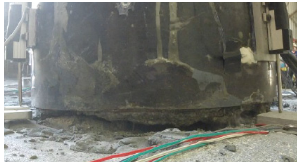
(b) South column interface, south side; \Delta = -7.5\%
