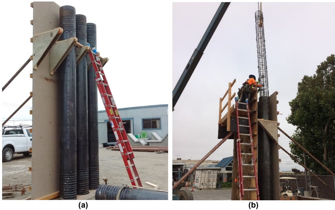
Figure 6.15 Concrete placing setup: (a) erect the column steel shells; (b) column reinforcing bar cages installation.
