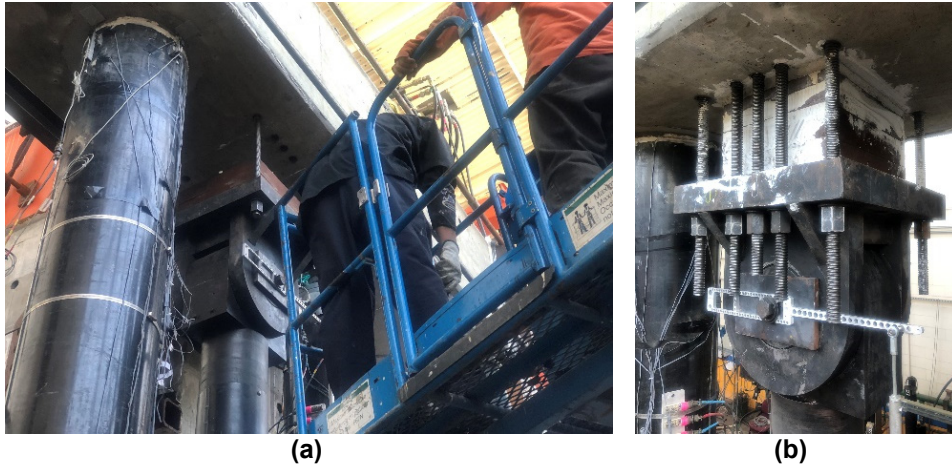
Figure C.12 (a) Install additional spacer plates to fill the gap between the vertical actuator and the cap beam; (b) extend the vertical actuator, grout the vertical actuator to the cap beam and install the vertical actuator connection rods.
