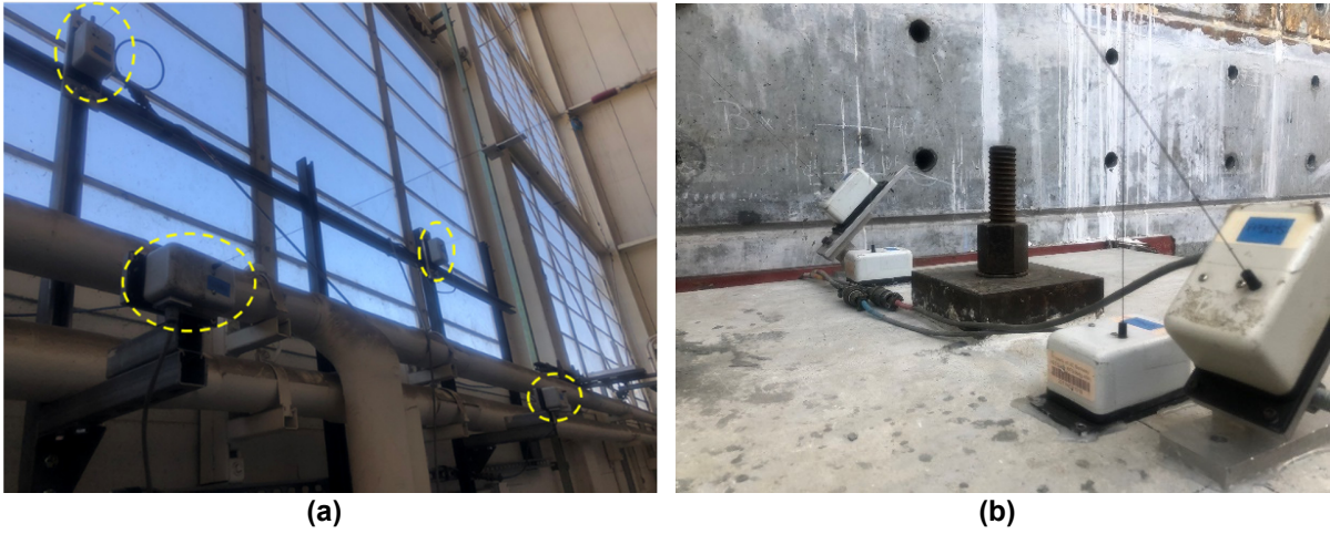
Figure 6.32 (a) WPs on the north-side instrumentation frame; (b) WPs between the cap beam and the foundation.
