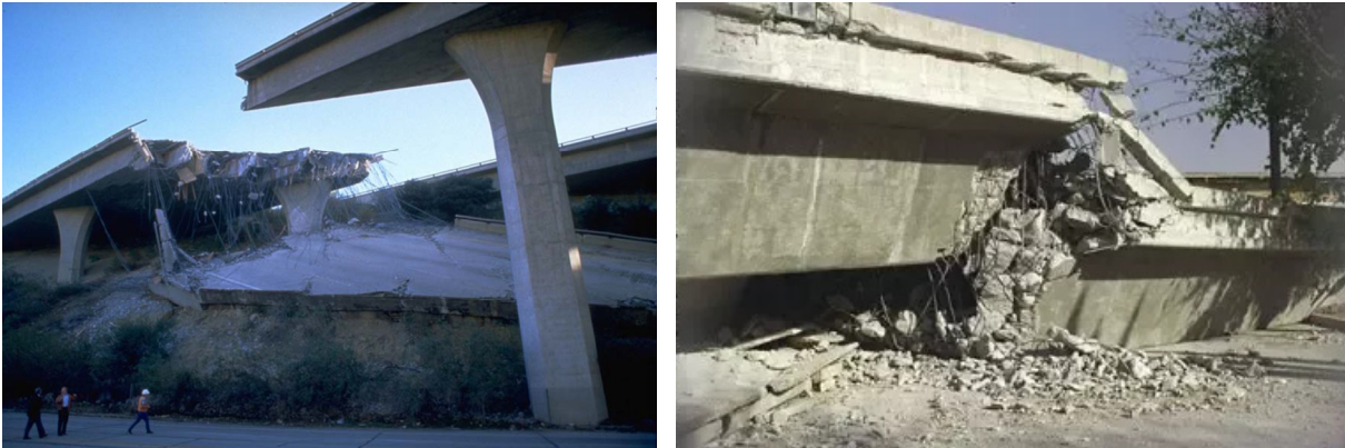
Figure 1.1 Damaged bridges after 1994 Northridge earthquake (source: FEMA photo library).
