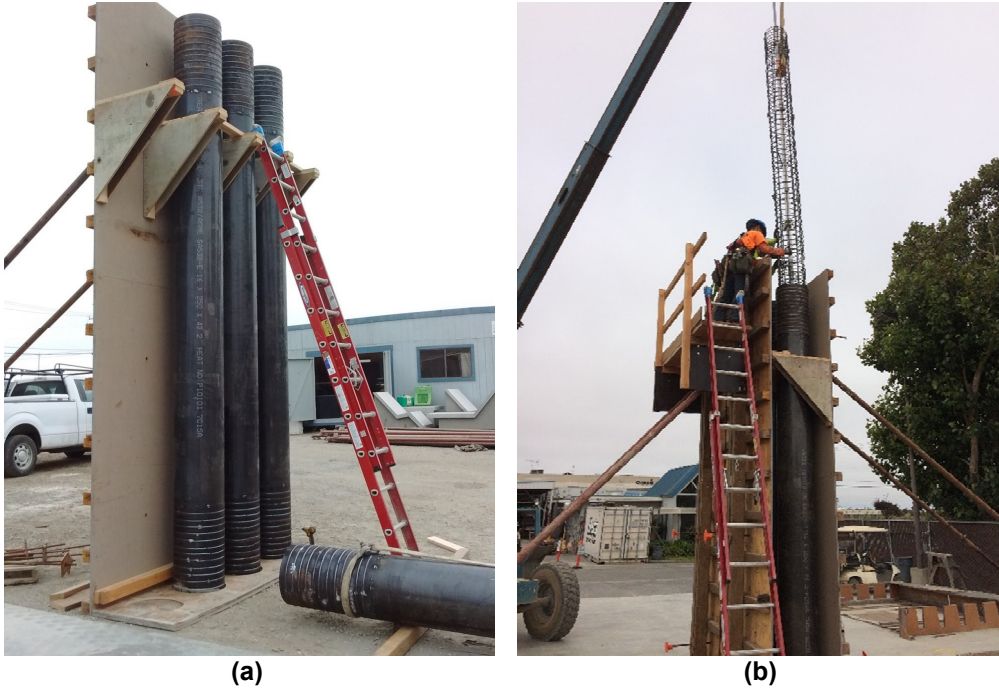
Figure B.4 Concrete placing setup: (a) erect the column steel shells as the permanent formwork; (b) column reinforcing bar cages installation.
