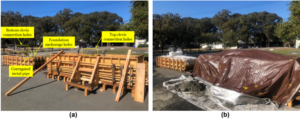
Figure 6.18 (a) Reinforcing bar cages and formworks before concrete casting; (b) concrete curing using curing blankets.
