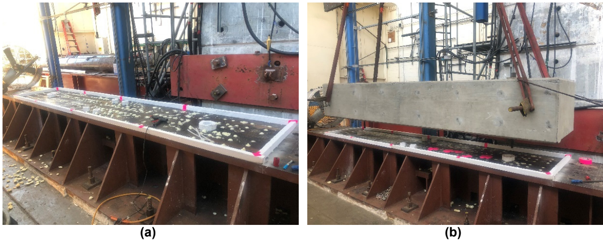
Figure C.1 (a) Prepare the surface and seal the holes in the supporting anchor beam; (b) lift up and install the foundation in place using the overhead crane.
