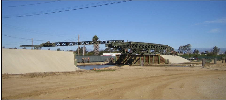
Figure 8-7 Photograph of the MGB with launching beam showing the bridge being pushed across the gap.
