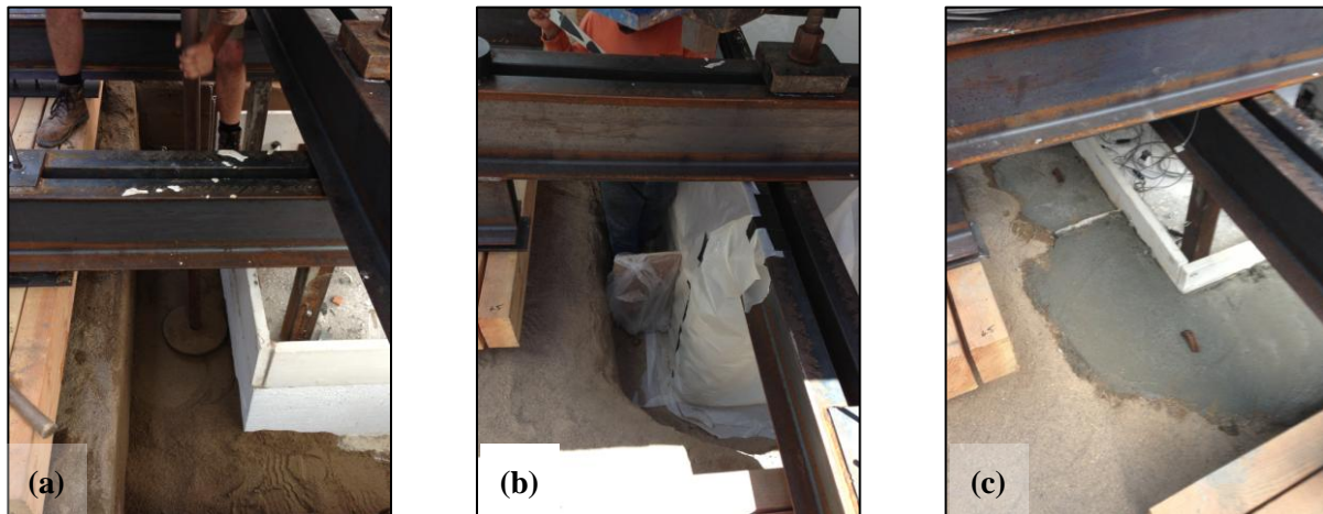
Figure 11. (a) Compaction by hand of the backfill sand for tests 1 and 2, and construction detail around the footings for test 3 (b) before and (c) after weak concrete casting.
