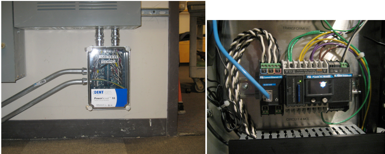
Figure 11: Left: Typical Dent installation. Right: One of two PSL PQube power meters.
