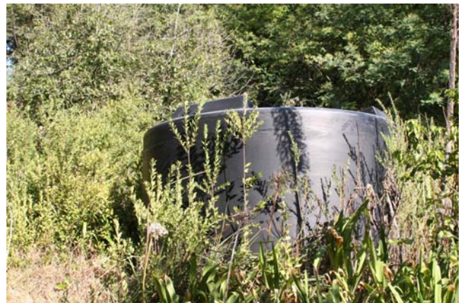
Figure 17: On-site Large Cistern approximately 1,600 gallons
