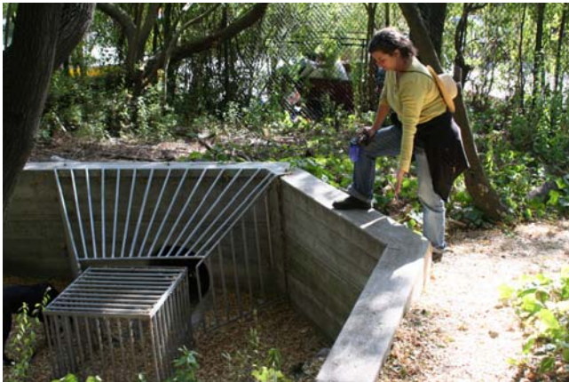
Figure 16: The creek goes into an underground culvert at the downstream end of the study reach
