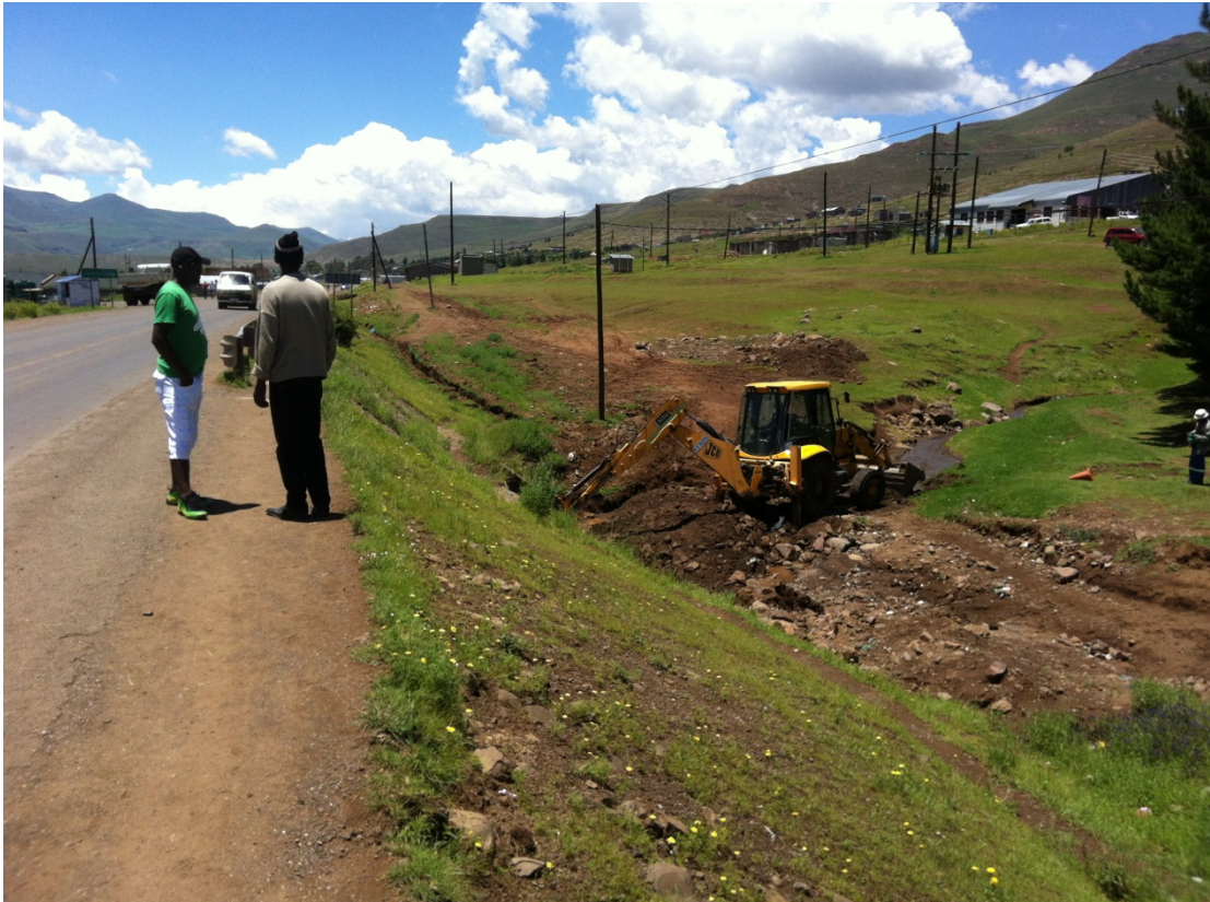
Figure 13: An excavator removes sediment blocking a culvert in Mokhotlong. Photo by the author.
