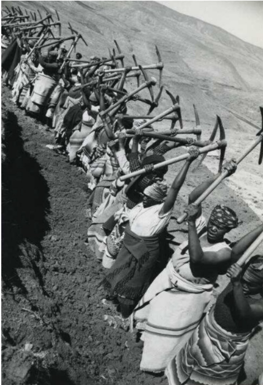
Figure 22: "Women comprise this work crew which is working on a cross-country road from east to west in Lesotho, ca. 1969" (photo by @marjmakh 2016).
