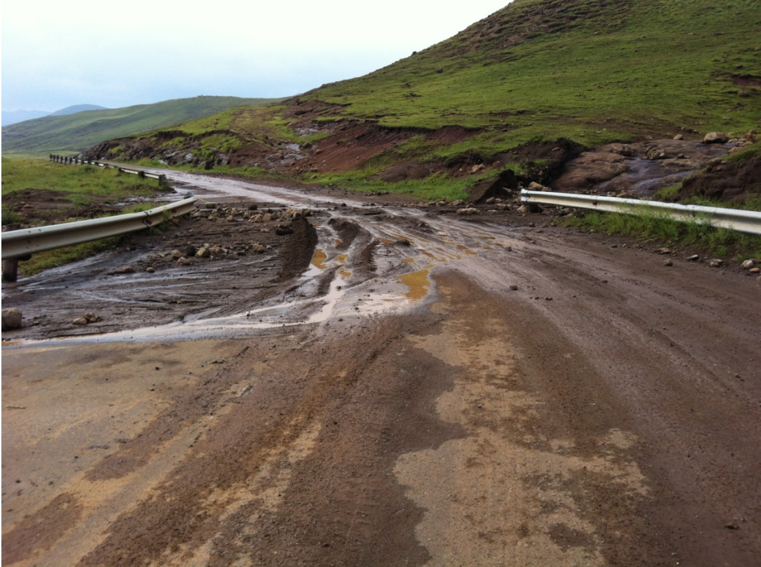
Figure 11: Road covered in sediment. Photo by the author.
