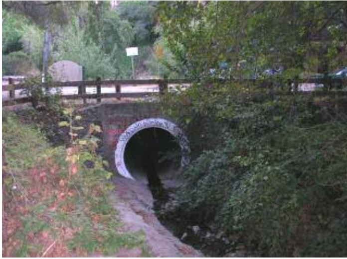
8a. Culvert at El Centro Avenue (View downstream, to the South North)
