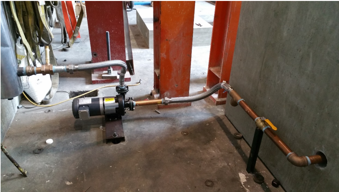
Figure 3.11. Heat transfer fluid tank heat circulation system.
