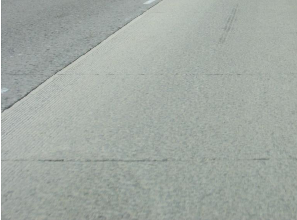
Figure C.2: Evidence of original longitudinal tines outside of the wheelpaths of Section QP-142.2 after one year of traffic.
