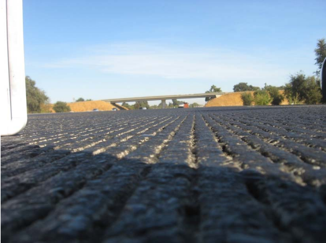
Figure A.10: Longitudinally tined, SI=105.5 dB(A) (Section QP-101.2).
