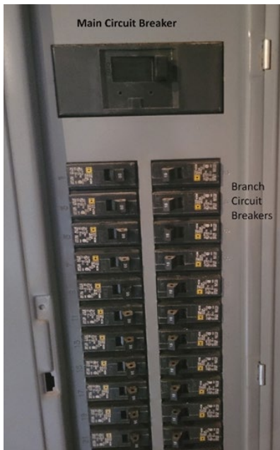
Figure 3. Example home breaker panel
