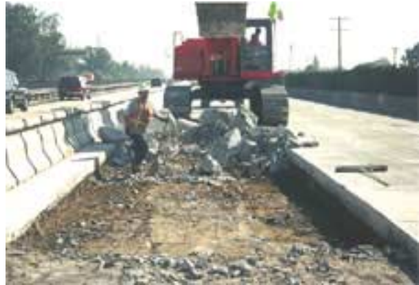
Figure 30. Removal of PCC slab, CTB, and part of aggregate base for full depth replacement.
