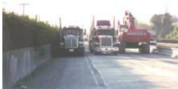
Figure 25. Excavator pausing operation to allow an end dump from other demolition team to pass.
