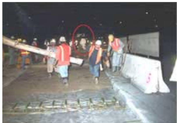
Figure 56. Cement ball from the mixer truck; evidence of buildup.
