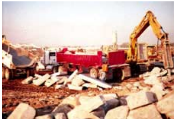
Figure 26. View of the dumping area with end dump trucks and breaker for rubblization.
