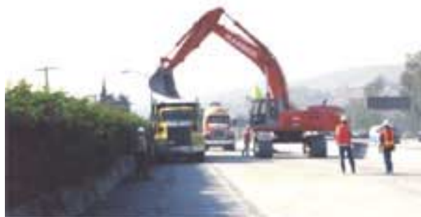
Figure 24. Concrete mixer truck waiting for clearance to pass behind the demolition operation.
