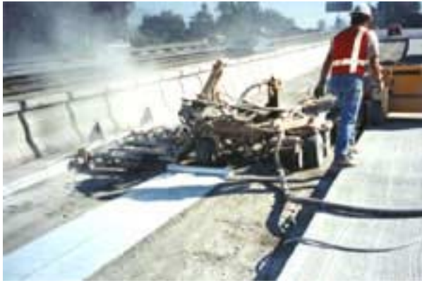
Figure 36. Self-propelled gang drill unit for drilling the bar holes to the existing slab.
