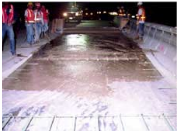
Figure 55. Example of poor quality, watery concrete.
