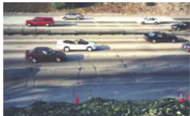
Figure 2. Typical failure of concrete pavement on U.S. Interstate 10.
