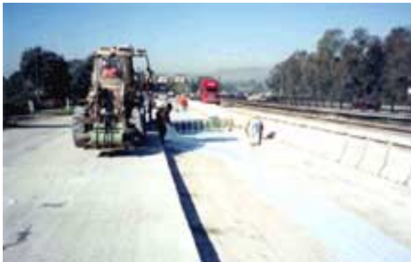
Figure 38. Placement of polyethylene sheet as a bond breaker between CTB and new slab.
