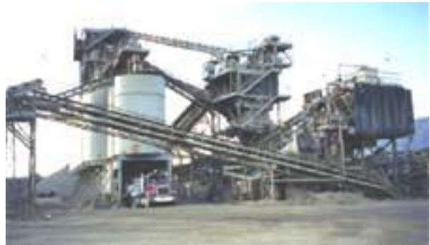
Figure 43. Vulcan Materials crusher plant (aggregate source).
