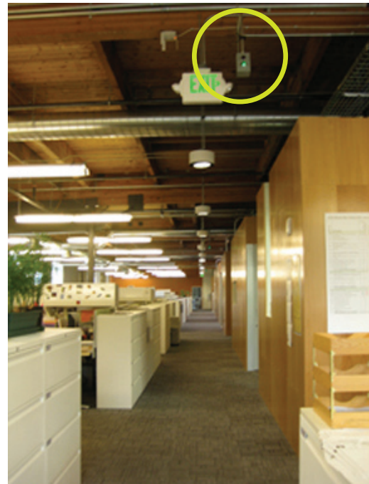
Red/green signals are located overhead in corridors, with other utilities
