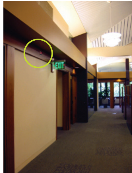
Signals are installed in the circulation areas between perimeter and core offices
