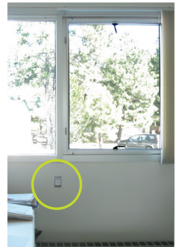
Signals are located below the window in each private office
