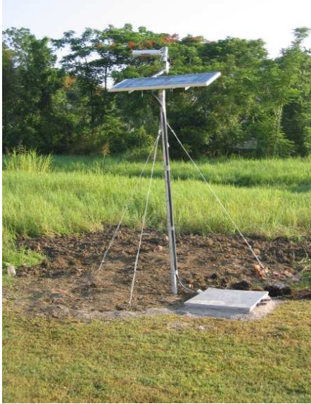
Figure 4: A single yagi antennae with solar panel and equipment vault at the HUEJ site.
