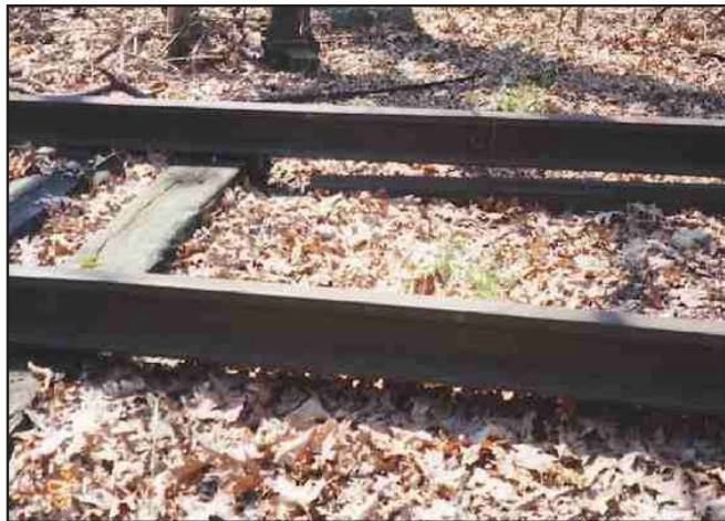
Photo 1. Observed under rail gaps at Nantasket Station. Woodlot Alternatives, 2003.
