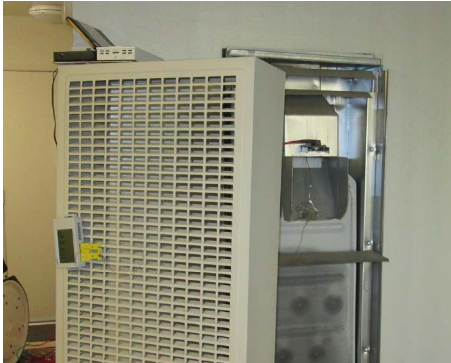
Figure 5. Placement of sensors around and inside a wall furnace.
