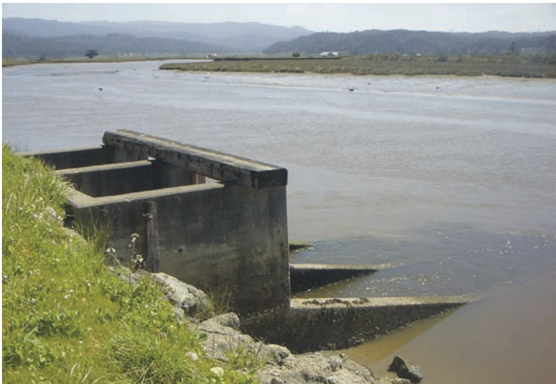
Figure 25. Tide gate separating Eureka Slough, Humboldt Bay, Humboldt County, California, and the drainage ditch that parallels California State Highway 101. Eureka Slough is in the background.
